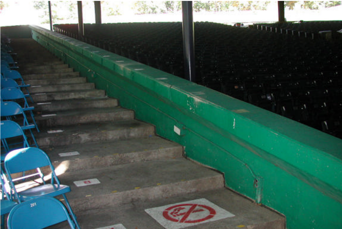
Original concrete cheek wall between original and added reserve seating on each side of Pavilion
