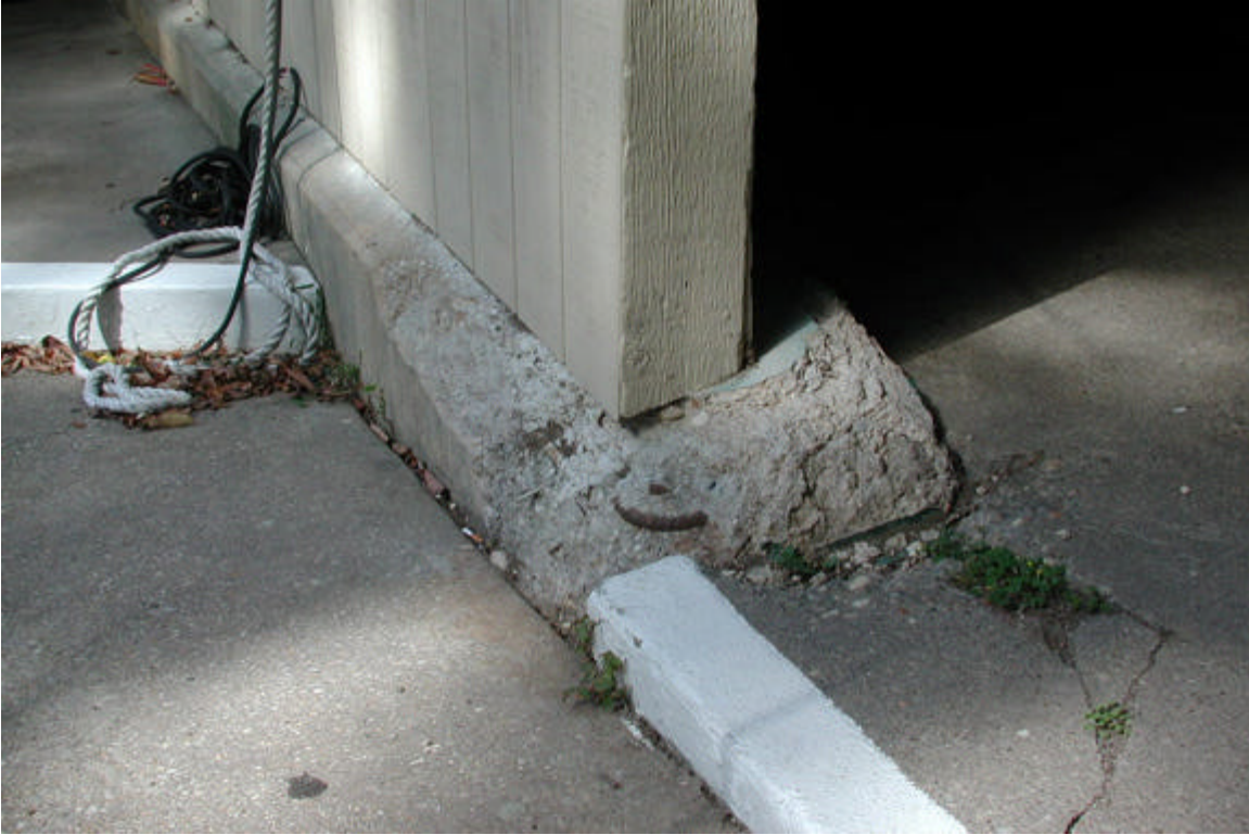
Characteristic concrete deterioration at Pavilion base, east side
