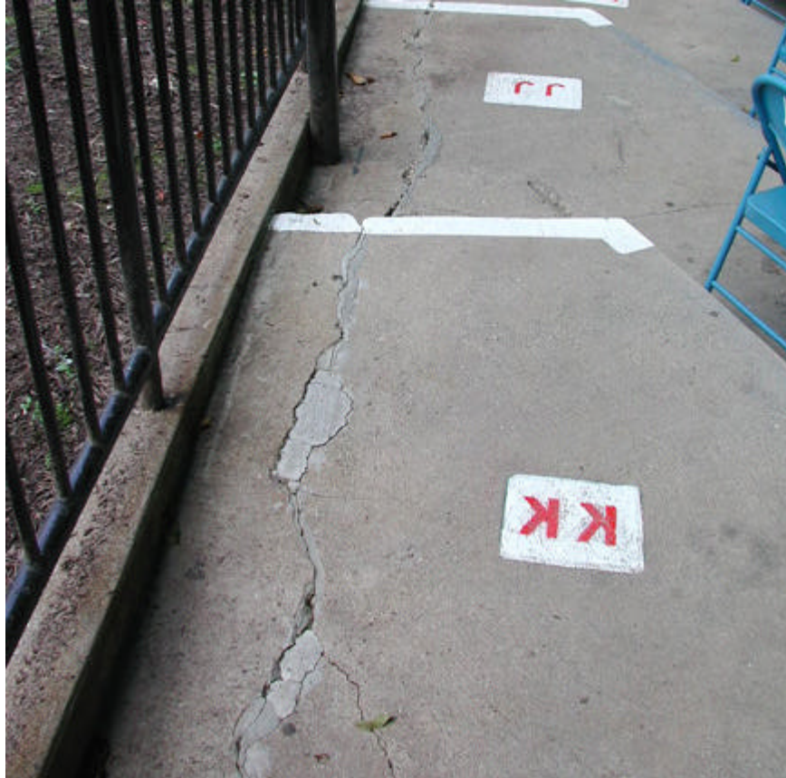
Characteristic settlement cracking at perimeter of West Loge
