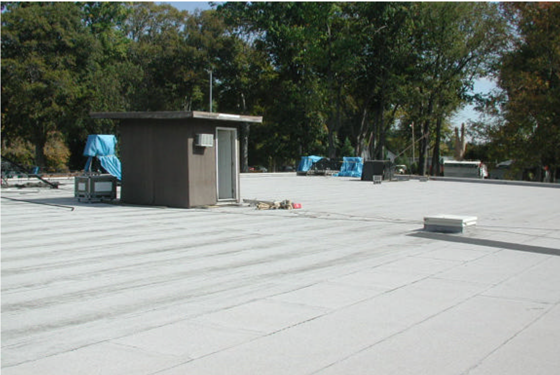
Roof showing access to follow-spot booth over center of reserved seating area
